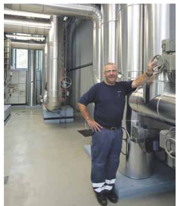
Boosterrum, Central Gimsing
